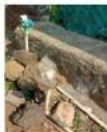
Fig. 12. Failed water pipeline
